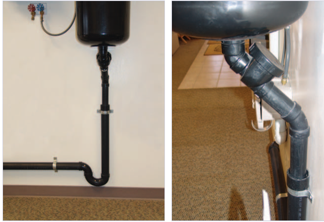
Flapper valve at 45° toward the wall, and the 1-1/2 in leg hanging loose in the 2 in standpipe.
